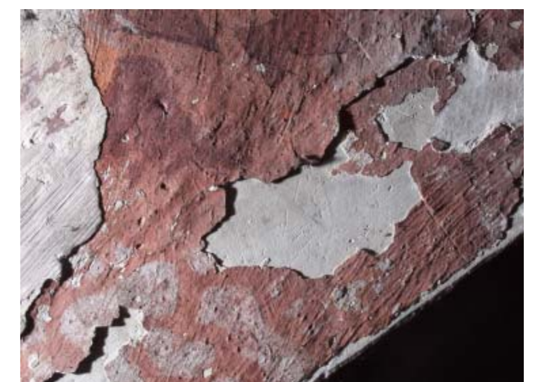
Delamination and flaking of the paint layer
